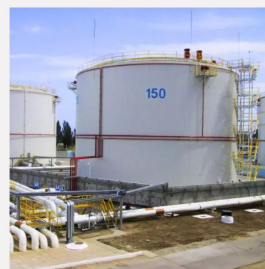
Tank Anticorrosive Coating
